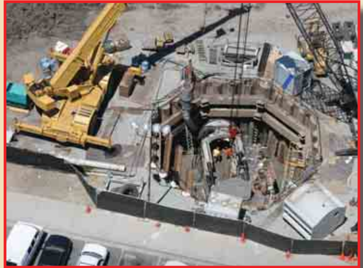
Aerial view of the octagonal launch shaft at Pacific Boring job site.
